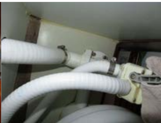
Manual pumps no leaks
