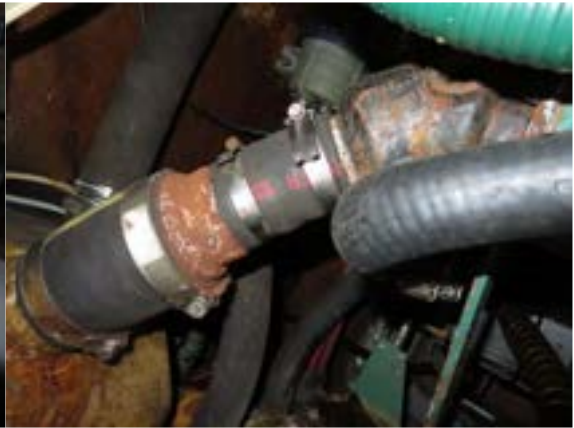
Exhaust intermediate connector corroded but no wastage
