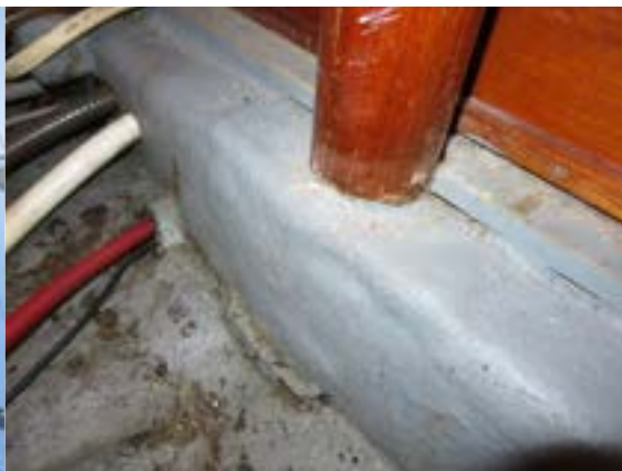
Laminations in way of mizzen compression post intact
