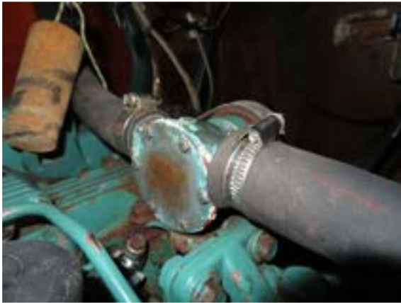
Impeller minor leaks only
