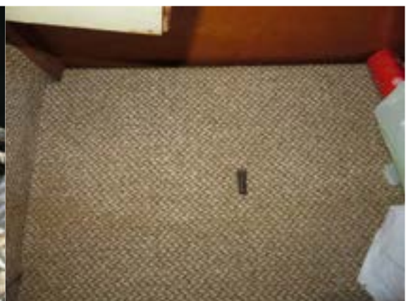
Hidden manual gas valve
