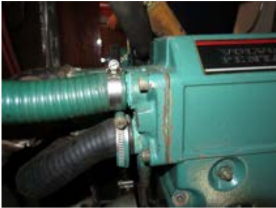
No leaks from heat exchanger
