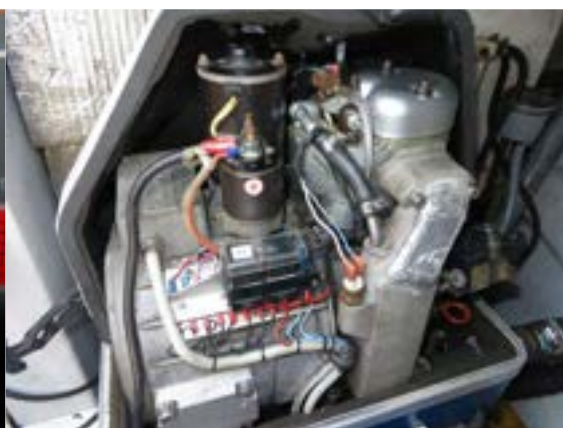
Generator without leaks
