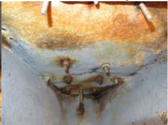
Anchor roller plate bolts corroded.
