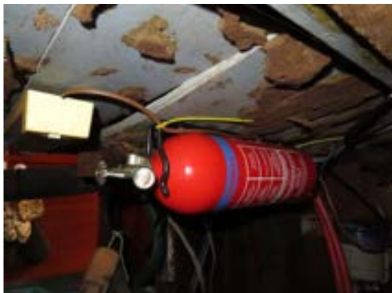
Engine room fixed firefighting installation
