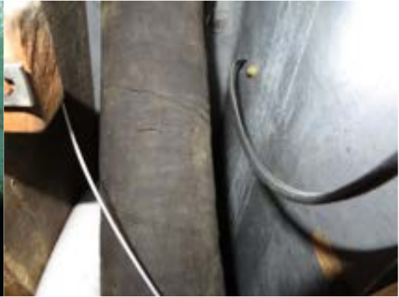
Exhaust hose with cracks
