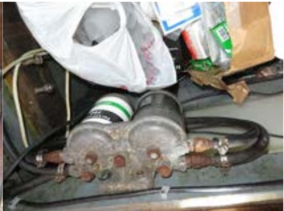
No leaks at filters
