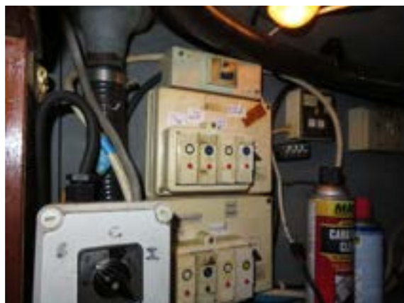
Shore power RCD
