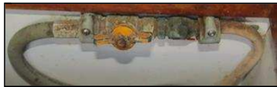
4.8 Item 3(Picture) LPG Cut off valve
