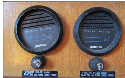
6.3 Item 2(Picture) High Water alarm in Bilges
