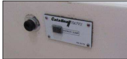
4.11 Item 2(Picture) Flush & sump pump
