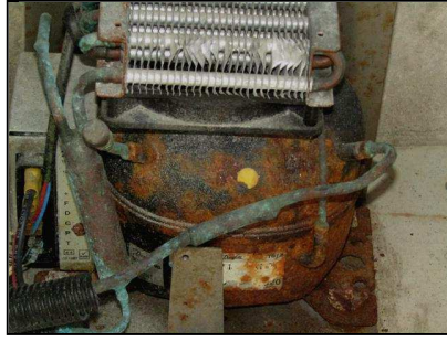
7.2 Item 1(Picture) Compressor after locker Compressor
