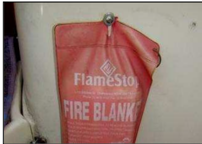
5.3 Item 1(Picture) Fire Blanket Fire Blanket
