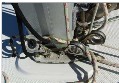
10.0 Item 3(Picture) Mainmast deck stepped Mainmast deck stepped c/w compression post inside accommodation
