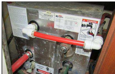
7.4 Item 1(Picture) HWS KUUMA 24 lt HWS 240 v AC and Heat Exchange off ME
