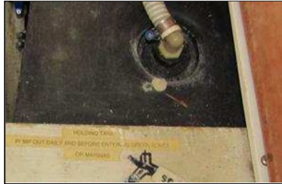
3.3 Item 1(Picture) Holding Tank Holding Tank under double berth
