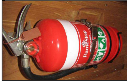
5.1 Item 1(Picture) DCP 1.0 kg FFE 1 - DCP in Hanging space in after cabin near Main Engine
