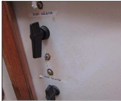
8.3 Item 1(Picture) Battery breaker switches
