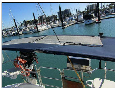
8.9 Item 1(Picture) Solar Panels
