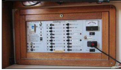
8.2 Item 1(Picture) Main Switchboard LH Side of Panel 240 v AC - RH side 12 v dc from ships power
