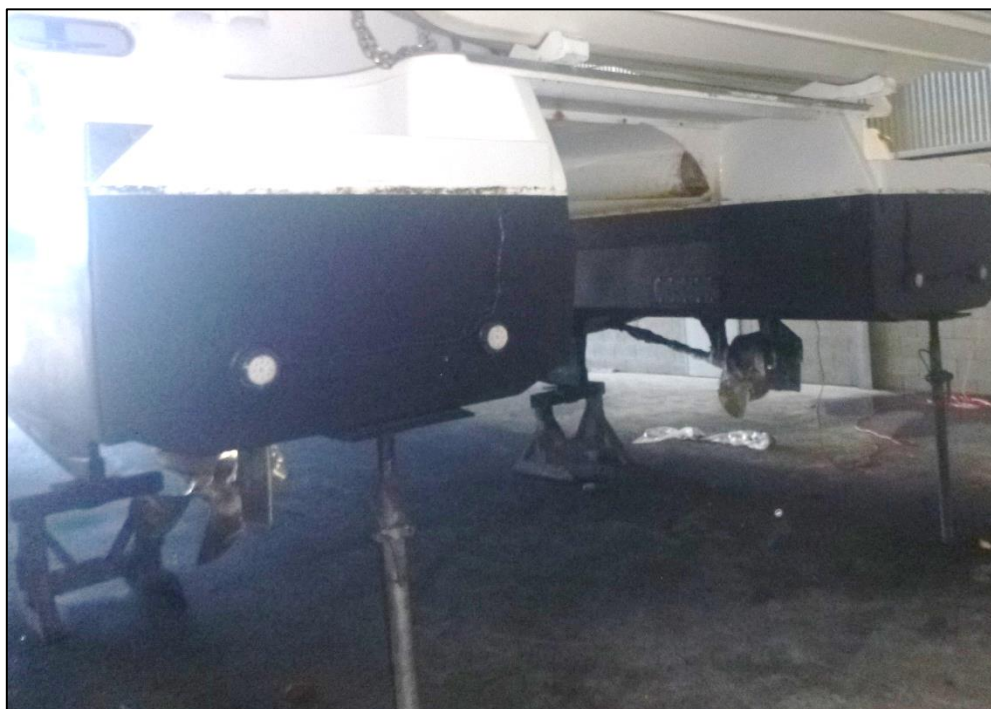
Running Gear – Pre Propspeed application
