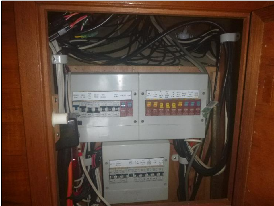
Electrical Management Board
