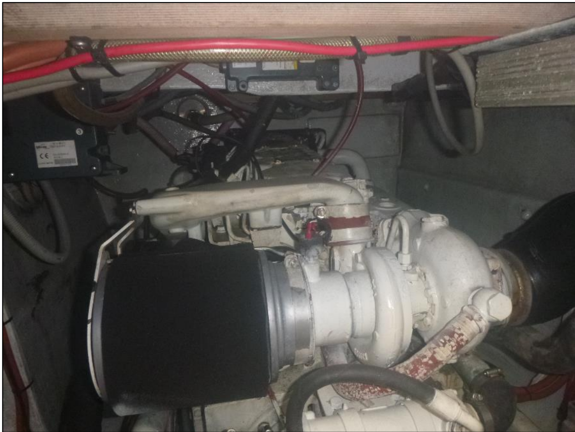
Starboard Main Engine
