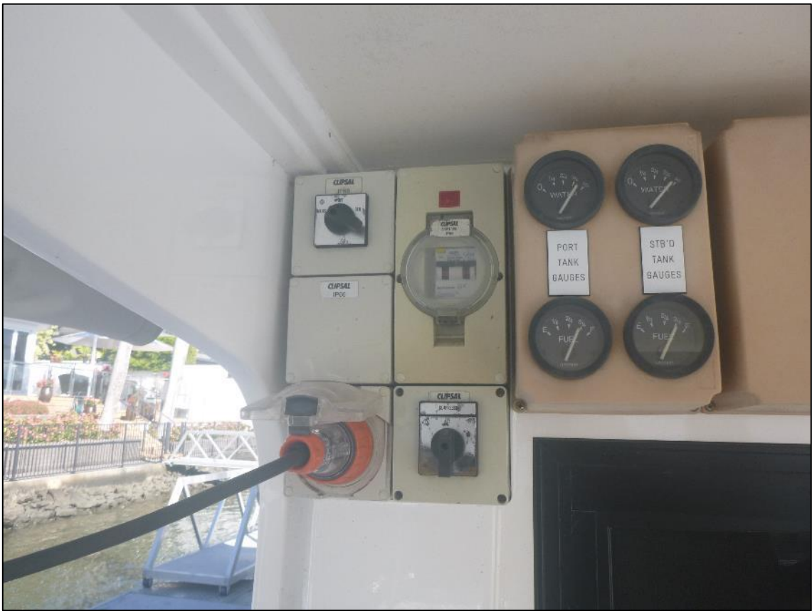
Shore Cable and Circuit Protection
