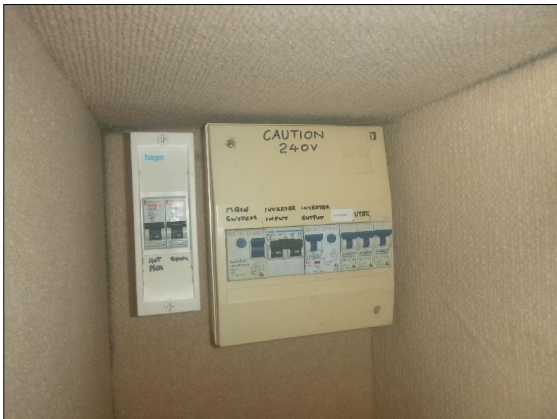
Electrical Management Board
