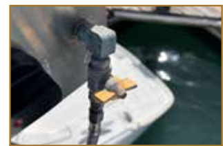
GAS ISOLATION VALVE
