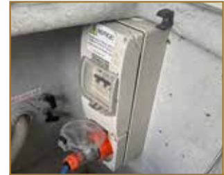
SHORE POWER CONNECTION
