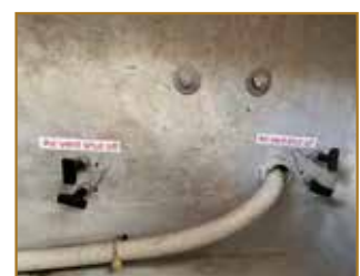
ENGINE ROOM AIR VENTS
