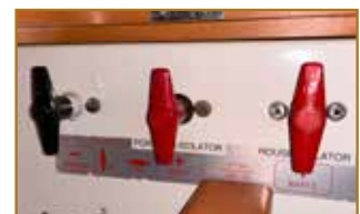
BATTERY ISOLATION SWITCHES
