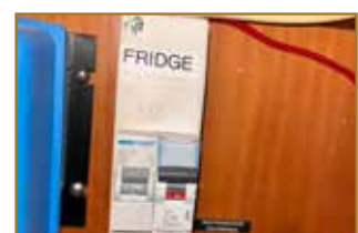
FRIDGE TRIP SWITCH
