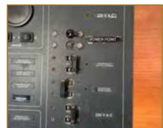
240V CIRCUIT BREAKERS
