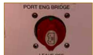
EMERGENCY BATTERY BRIDGE SWITCH
