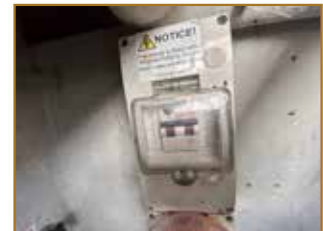
SHORE POWER CIRCUIT BREAKERS
