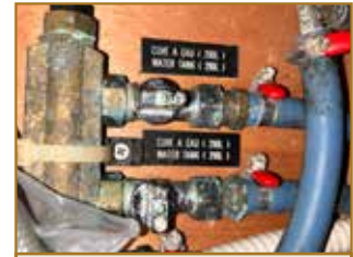
WATER CHANGEOVER VALVES
