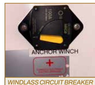
WINDLASS CIRCUIT BREAKER
