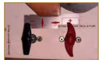
BATTERY ISOLATION SWITCHES
