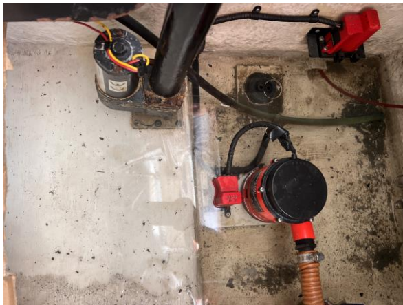
Engine Room Bilge
